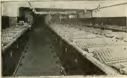
STORAGE BATTERY ROOM.
